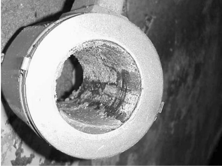
FIGURE 10.9 Struvite deposits found in 75-mm (3-in.) magnetic flowmeter on dewatering centrate line. The thicker the deposit on the flowmeter, the bigger the error because the meter measures more flow than is actually there because of the reduced diameter.
