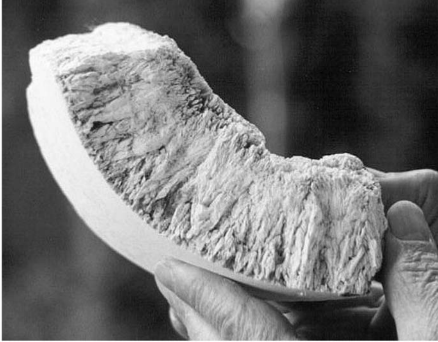
FIGURE 10.8 Struvite deposit from a 0.3-m (12-in.) lagoon decant line, which broke loose and got caught in a check valve at Columbia Boulevard Wastewater Treatment Plant, Portland, Oregon.
