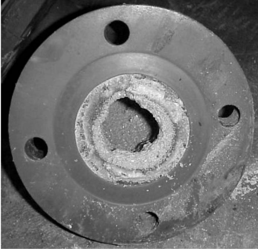
FIGURE 10.13 Struvite deposits in a 75-m (3-in.), rubber-lined, 90-deg elbow; the buildup occurred during a two-month material testing period.
