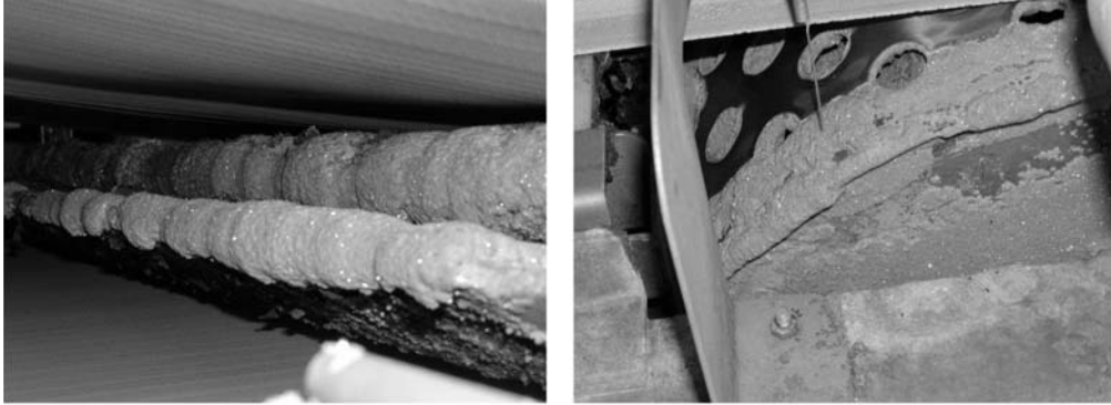
FIGURE 10.15 Struvite deposits on a belt filter press.
