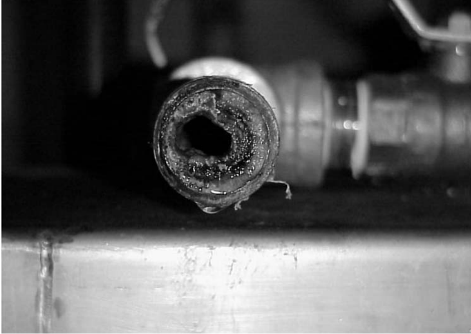
FIGURE 10.10 Image of struvite deposit in 25-mm (1-in.) pipe to a streaming current meter, which controlled dewatering polymer feed. Inaccurate measurement by the streaming current meter, as a result of the deposits, can result in polymer overdosing or reduced dewatering performance.
